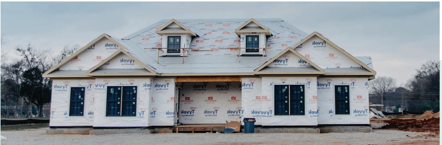
A duplex is also in construction to benefit our college students, missions teams, and off-duty house parents.
